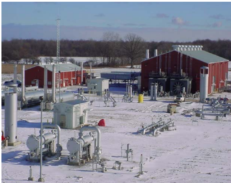
Transmission and Storage Compressor Station Sempra Gas Columbus, MI
